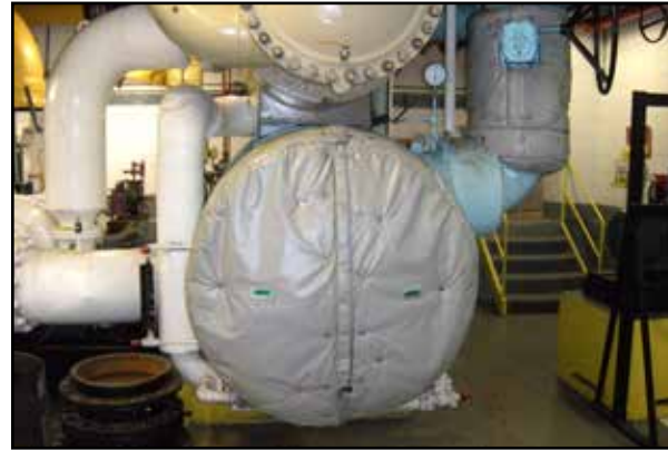
LT250VP CHILLED WATER HX HEAD & VALVES
