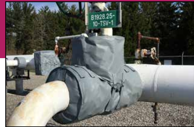
SSS-500-TAFT OIL PIPELINE - SHUT OFF VALVE
