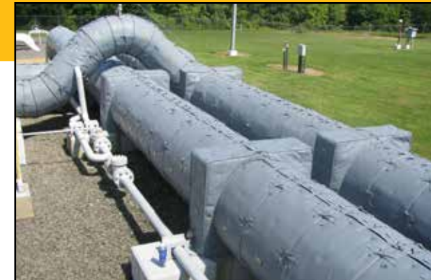
LT450A-TT NATURAL GAS PIPELINE 24" (13 dBA REDUCTION)
