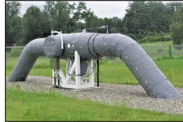
LT450-HES NATURAL GAS PIPELINE
