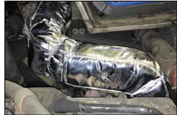
HT1300AGM EXHAUST ELBOW & PIPING
