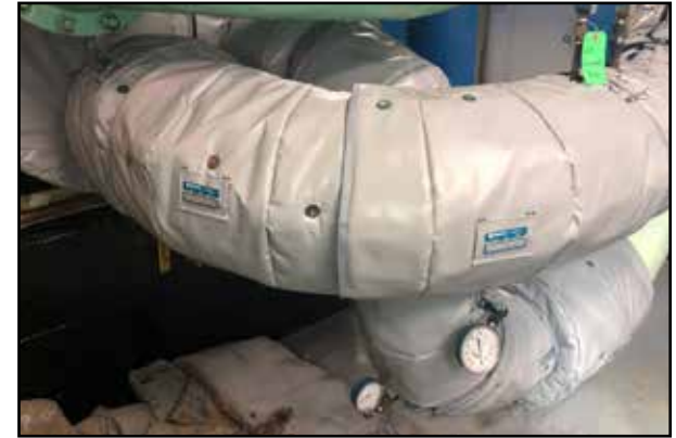
LT250VP CHILLED WATER VALVES & PIPING
